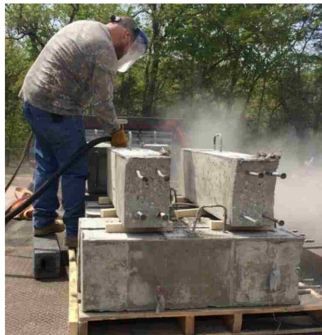
(d) Figure 3.7 Figure showing various surface preparations (a) smooth/ no-surface (b) roughening (c) sandblasting (d) technician preparing beam-joint interface at Missouri S&T mines
