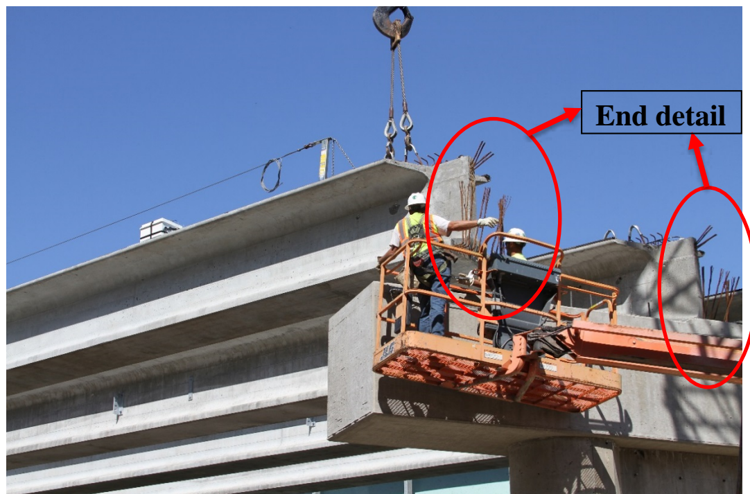
Figure 2.13 Girder erected in position for Highway 50 Bridge with MoDOT end girder detail
